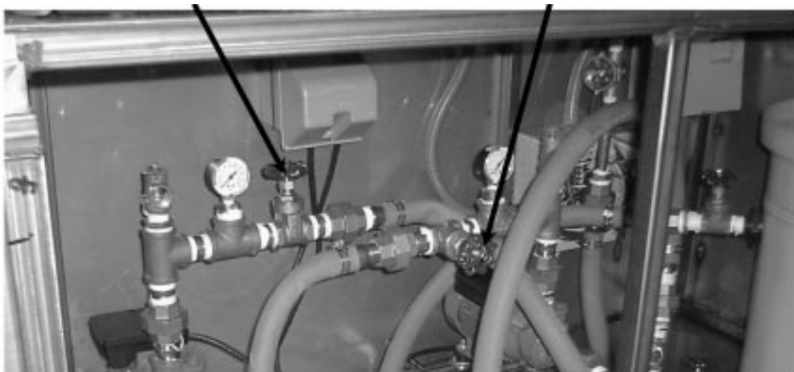
Fig. 7. Flow control valves.
