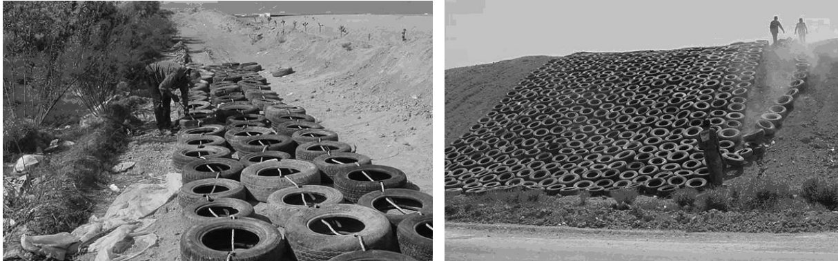
Fig. 3. Insertion of an anchored rope through the tires (left) to build the lines that will cover the slope (right).
